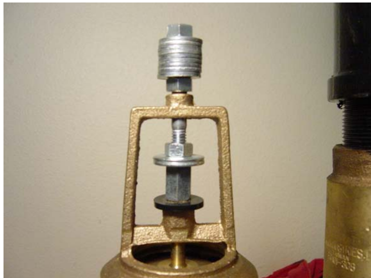
Conversion to Waste / Impetus Valve complete
