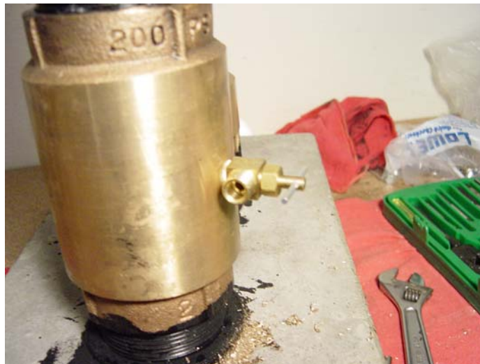
Needle valve installed.
